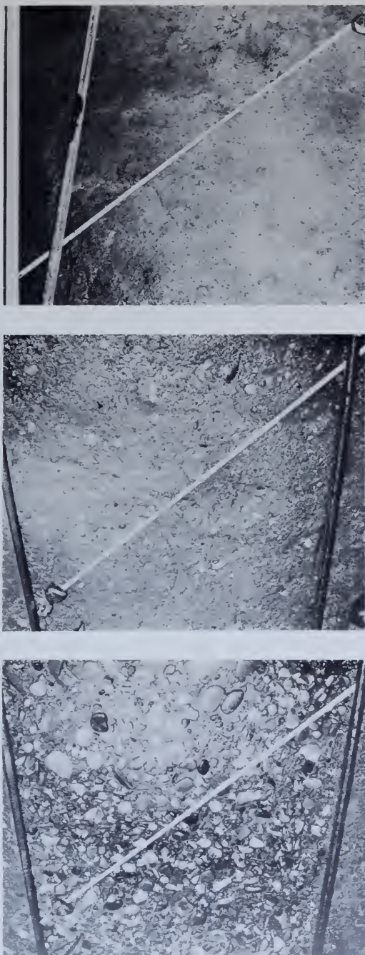
Figure 125.—Comparison of construction joint treatments. Top: construction joint surface before sandblasting. Middle: after correct sandblasting. Bottom: after oversandblasting, causing aggregate to be undercut. PX-D-33033.
